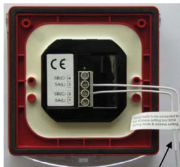
Flying leads to be connected to the address setting tool 3314/4414 during mode and address setting
